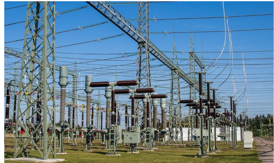
Figure 13. High-voltage electrical substation
