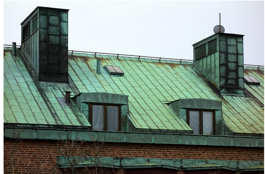
Figure 17. Copper roofing and rainwater system
