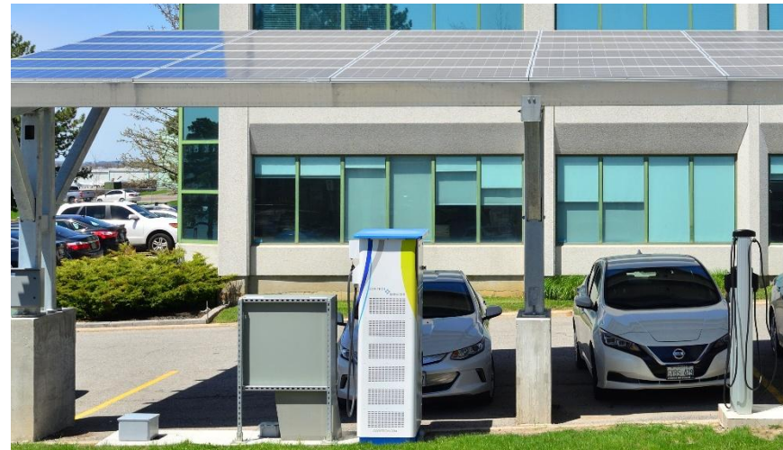
Figure 24. Electric vehicles charging at a solar-powered EV charging station
